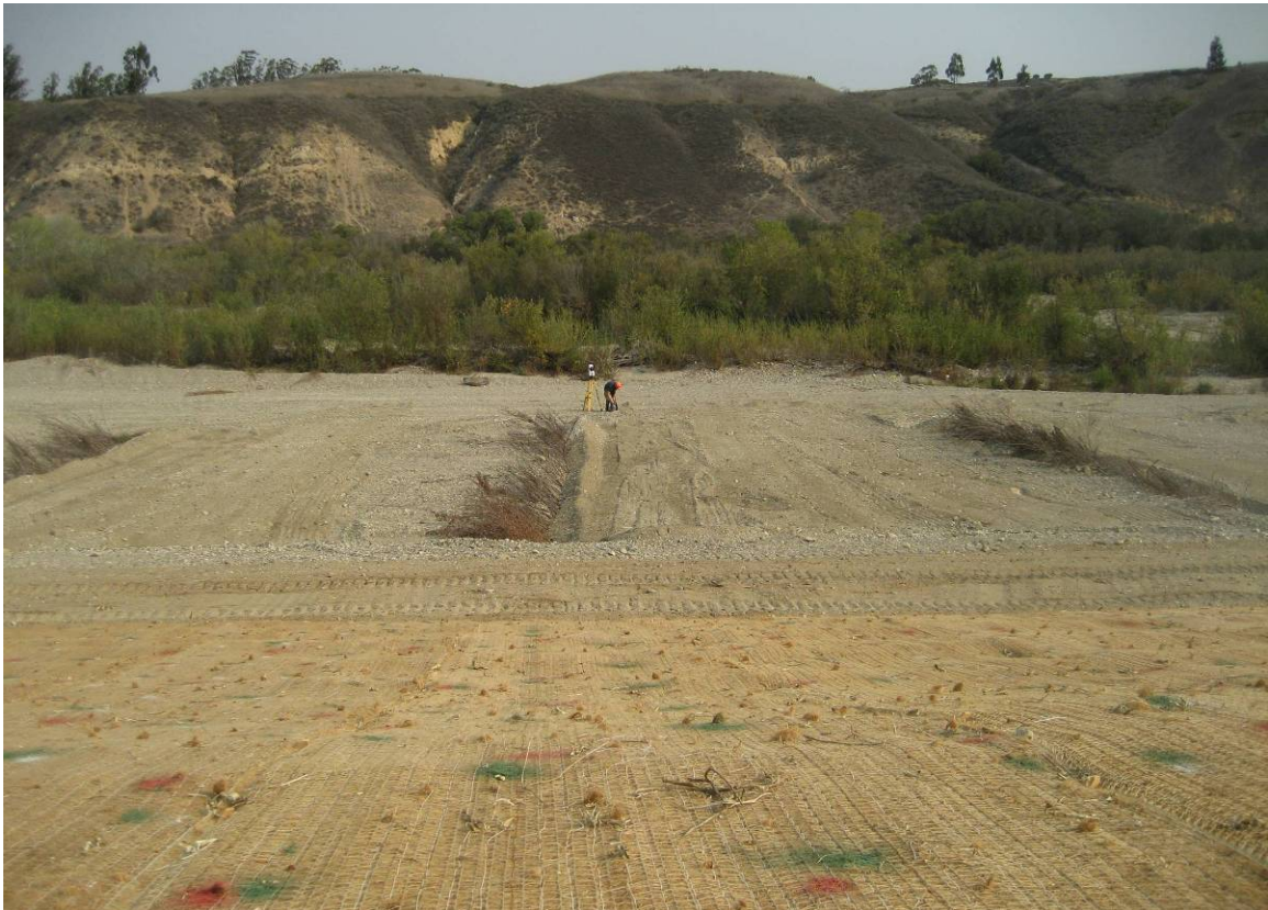
Figure 48: The as-constructed coir-fabric stabilized 2:1 slope, the (un-vegetated) relief terrace, and the willow baffle rows.
