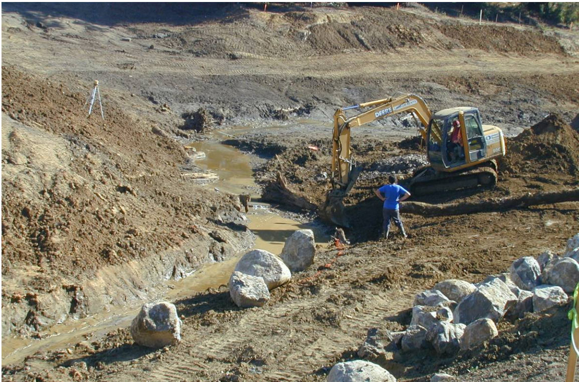
Figure 23: Installation of boulder and large woody debris features in the new channel.
