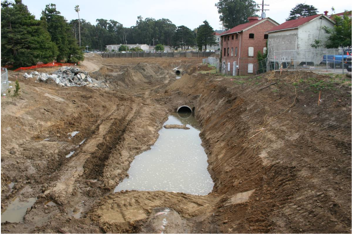
Figure 20: The culvert previously containing the Tennessee Hollow creek was removed during site grading. Temporary dewatering operations were required.
