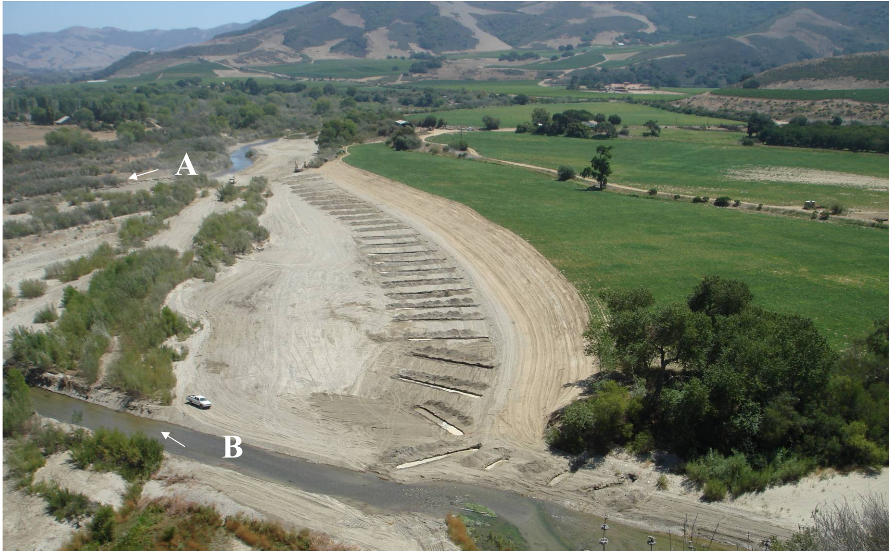
Figure 44: A view looking upstream with grading of the river bank in progress and excavations for the willow baffles is in progress. Photos from locations “A” and “B” are shown in Figures 45 and 46, respectively. Photo by Meredith Hardy.
