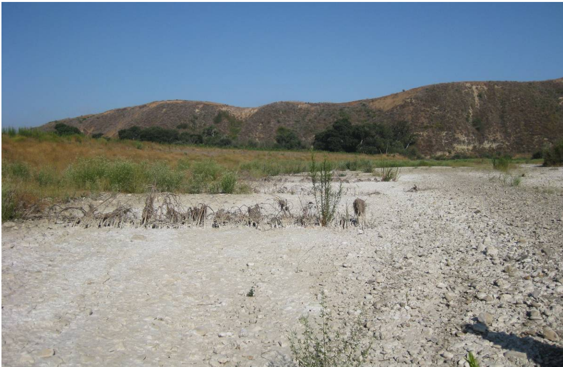
Figure 54: A view (downstream) of willow baffle segments damaged by the winter flows that ‘jumped’ the temporary bypass channel.
