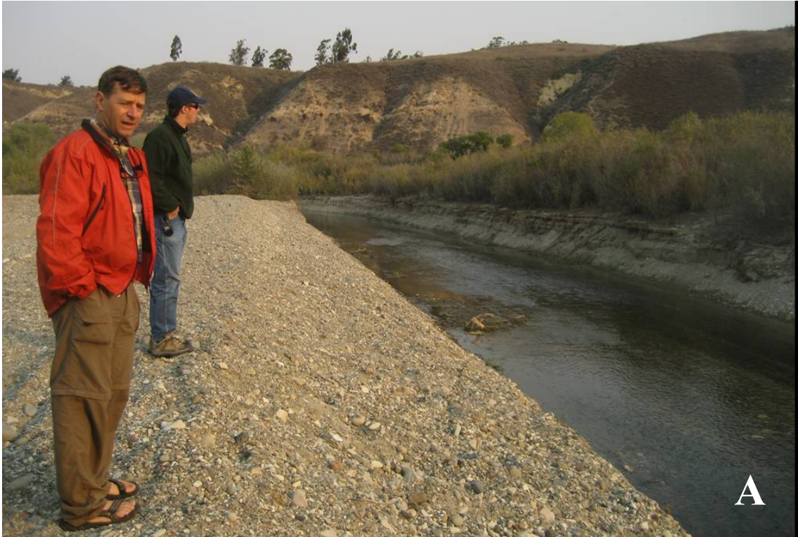
Figure 45: The upstream start (location A) of the temporary bypass channel installed to divert flows during construction and for the first several years after construction to allow the bank stabilization vegetation time to establish.
