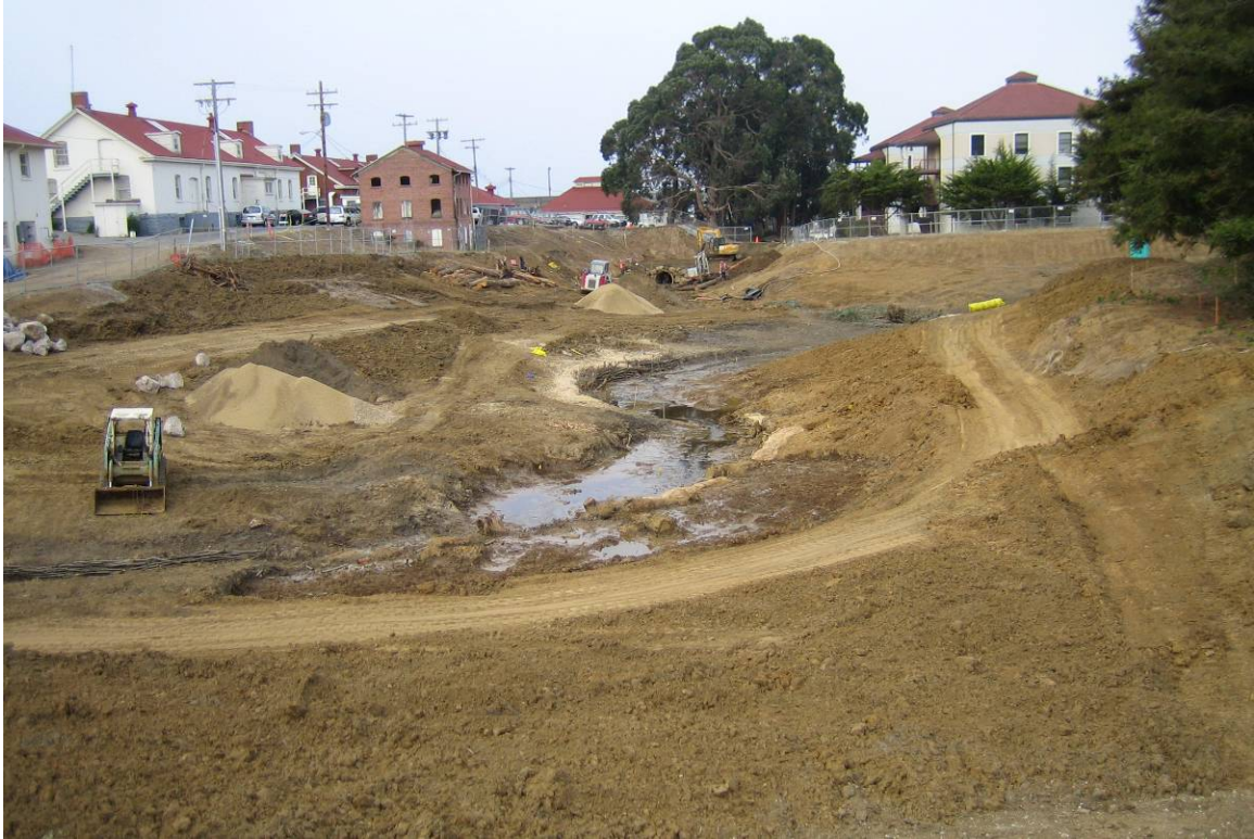
Figure 22: A northward view of the restoration near the end of earthwork operations shaping the new creek channel.
